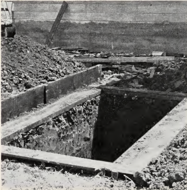
Fig. 5—Rectangular frame about the hole. The 2 × 10-inch planks are later used as baffle boards.
